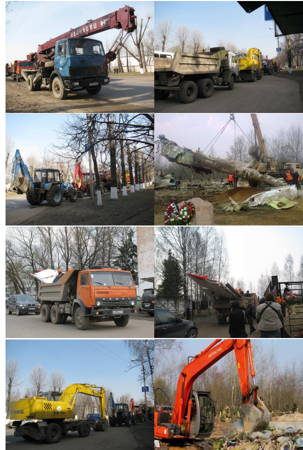
Figure 17: Some of the heavy equipment operating on the crash scene on April 11-14, 2010, on the crash site by Dr. Jan Gruszynski.
